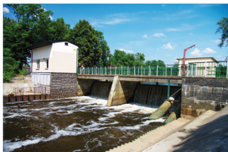
→ HYDROELECTRIC POWER PLANT ON THE LIWIEC RIVER → photo: Grzegorz Hubert Gerek
